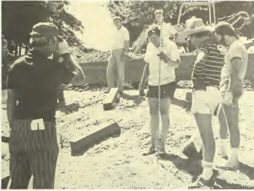
Under the Adopt-A-Park plan, industry lends a helping hand to the residents of the Easy Bay. Here executives and employees of Kaiser Aluminum & Chemical Corporation help put together a playground for Roberts Recreation Area.
