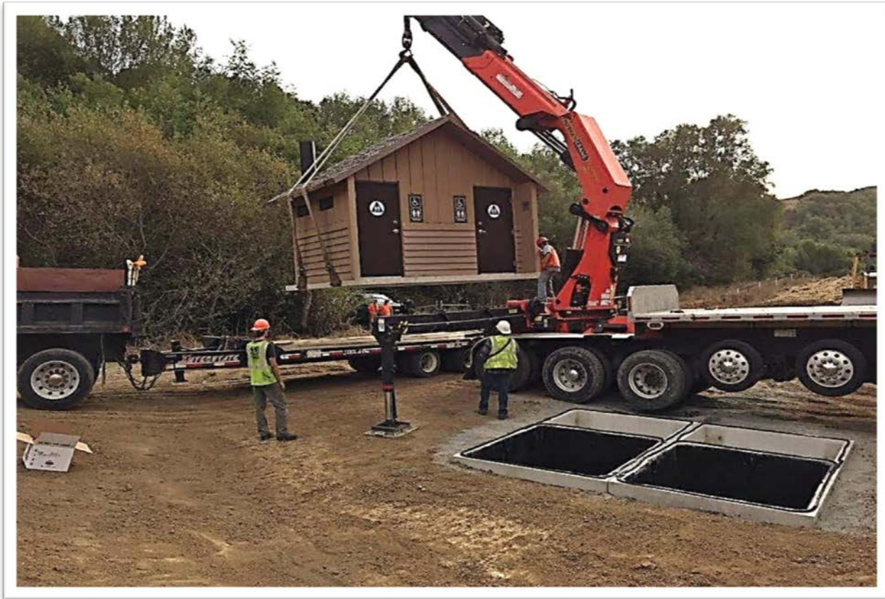
Installation of the CXT restrooms for the Wee Ta Chi group camp
