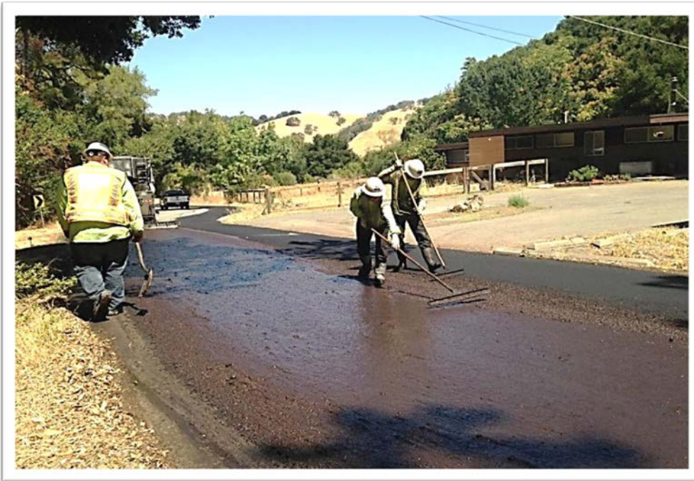
Photo above shows the two step application of the fiberized micro surfacing process. The process involves mixing shredded fiberglass in the slurry sealing process.
