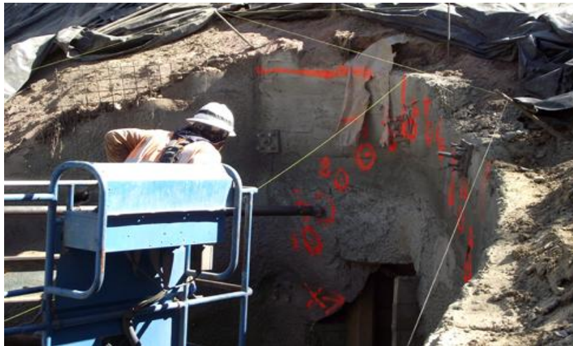
The replacement of the Greathouse Portal is underway (above); the portal serves as the entry to the mine's visitor center.
