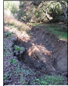
31 Deteriorated culverted channel in proposed Alder Creek restoration area in McCosker sub-area
