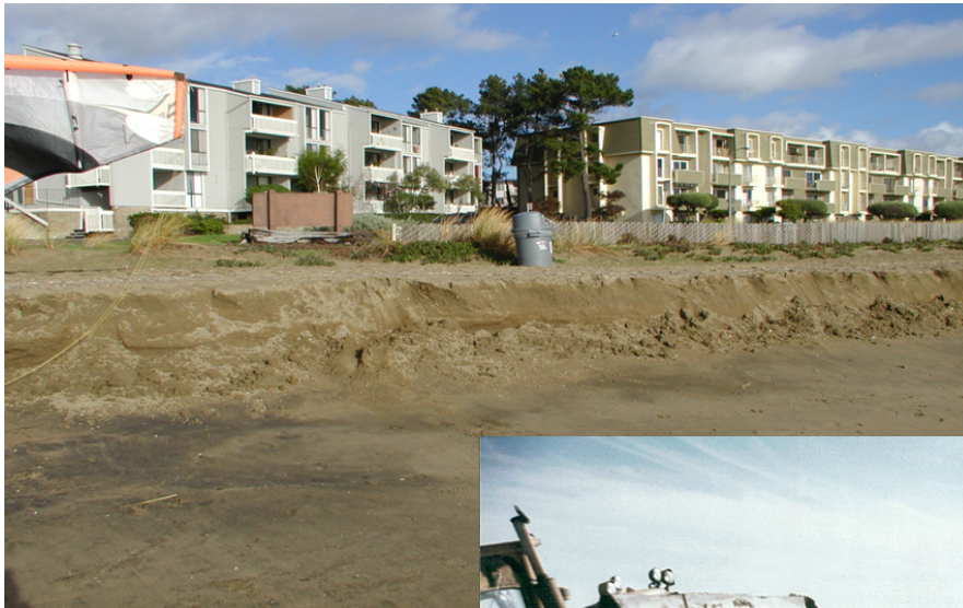
The photo on the left shows sand erosion at Westline and Shoreline drives.
