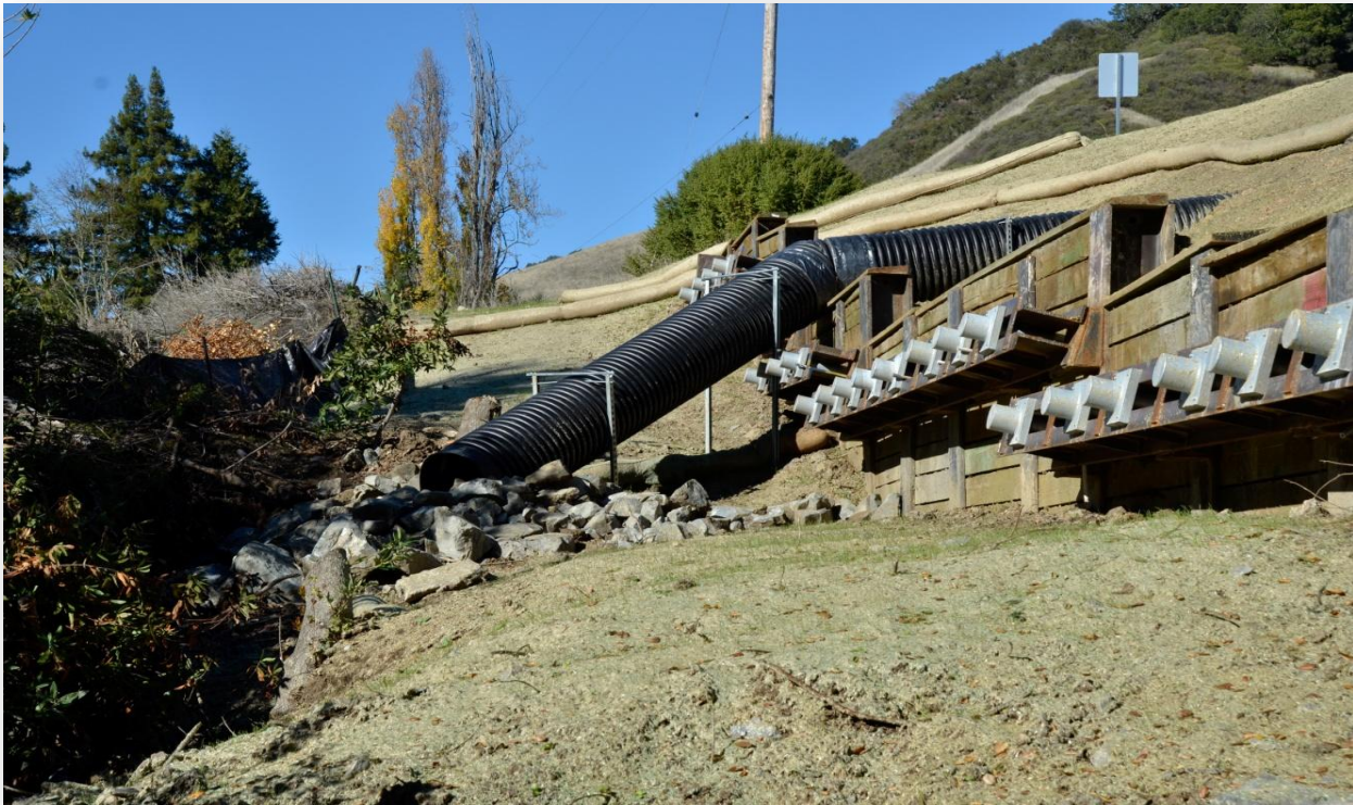
Rods were drilled into the slope and grouted in place as part of the anchoring system for the retaining wall.
