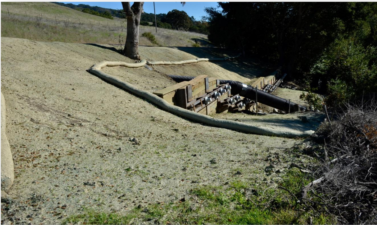
Repair of this landslide on Bollinger Canyon Road at Bollinger Creek restored the full road width to public access and protects the creek bank.
