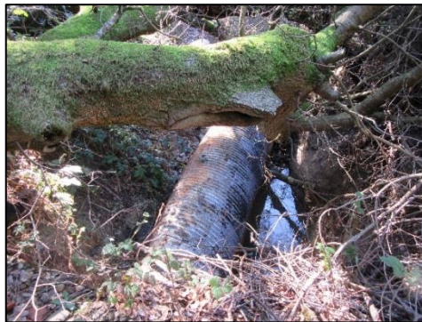
30 Deteriorated culverted channel in proposed Alder Creek restoration area in McCosker sub-area
