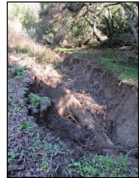
31 Deteriorated culverted channel in proposed Alder Creek restoration area in McCosker sub-
