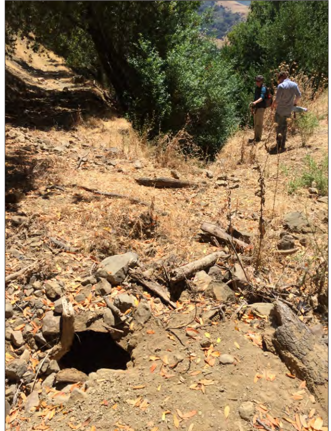
Photo 12 - Road damage requiring stabilization of trail with culvert upgrade and head/tail walls (Improvement #10).
