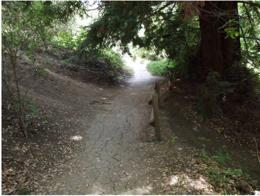
Location 5: 3rd split-rail fence upstream from Nook Pool (at large Redwood tree). Here water erosion from the opposite of the trail is evident. A retaining wall could be effective for reducing the amount of erosion entering Wildcat Creek.
