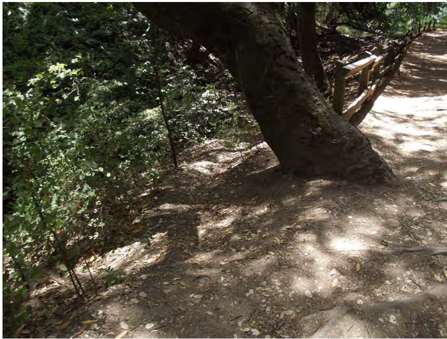
Location 2: 1st split-rail fence after Nook Pool (upstream). Here you see an obvious bootleg path leading to the creek. Fencing should be extended here to deter hikers and dogs.
