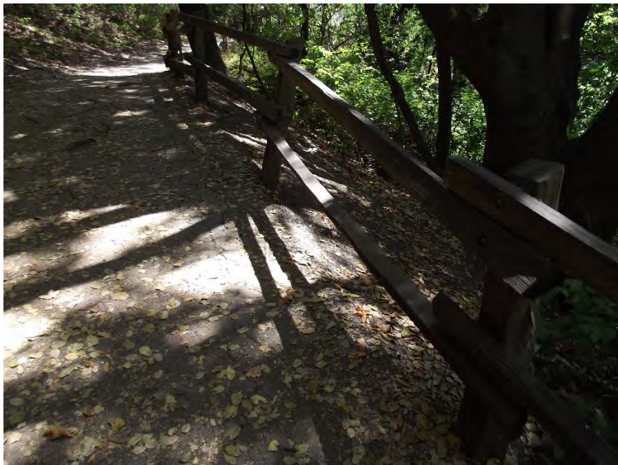
Location 11: 1st split-rail fence upstream from bay trees at large bay tree. Water erosion is again evident from opposite side of trail. Re-vegetation or a retaining wall is recommended.
