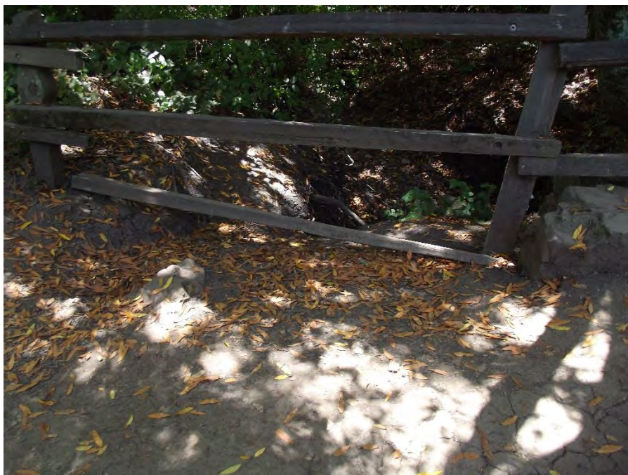
Location 7: Stone culvert. This site is also experiencing erosion from water runoff which is draining directly into a tributary. A retaining wall is recommended.
