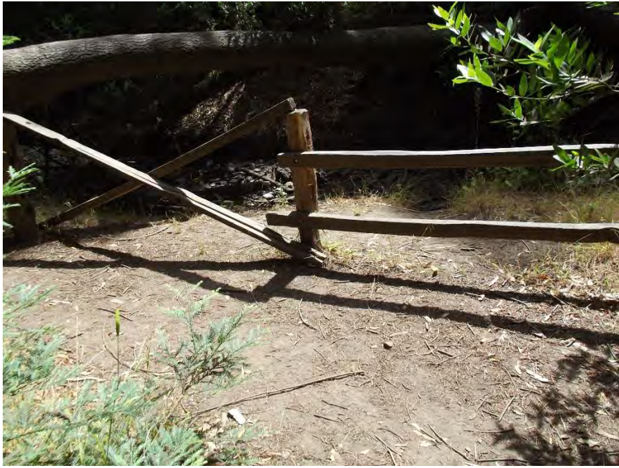
Location 14: End of split-rail fence near 2 large Redwoods. Fencing is in need of repair and netting installed. This area is extremely close to the creek and is very easy to access.
