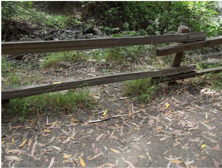
Location 18: Alternate view showing the need for mesh on bottom of fence.
