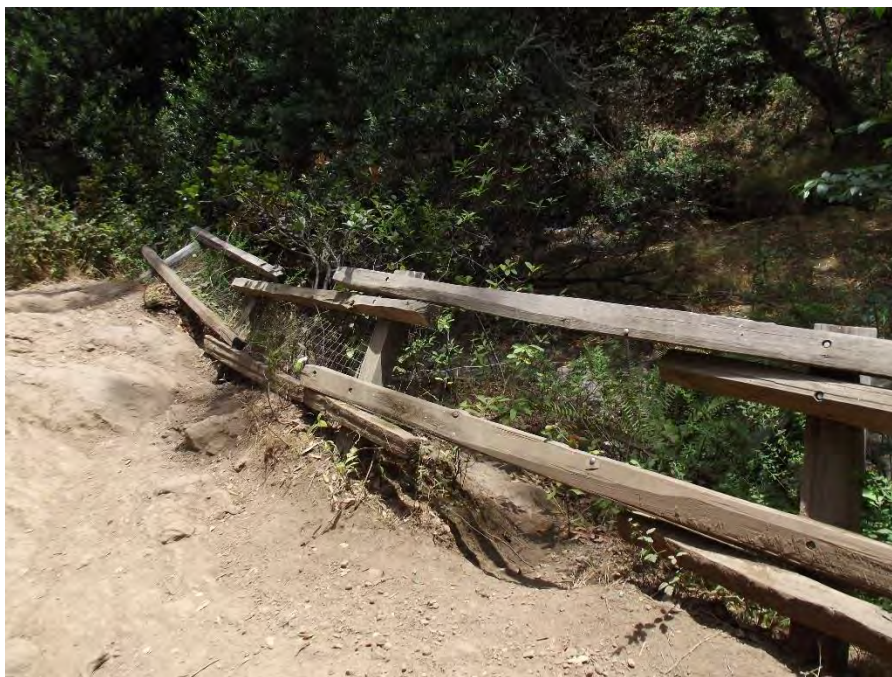
Location 1: Nook Pool. Further up the trail, this fence is falling over and in need of repair. Also netting should be placed at the bottom of the fence. This was the second most popular entry location for dogs entering Nook bank and pool.
