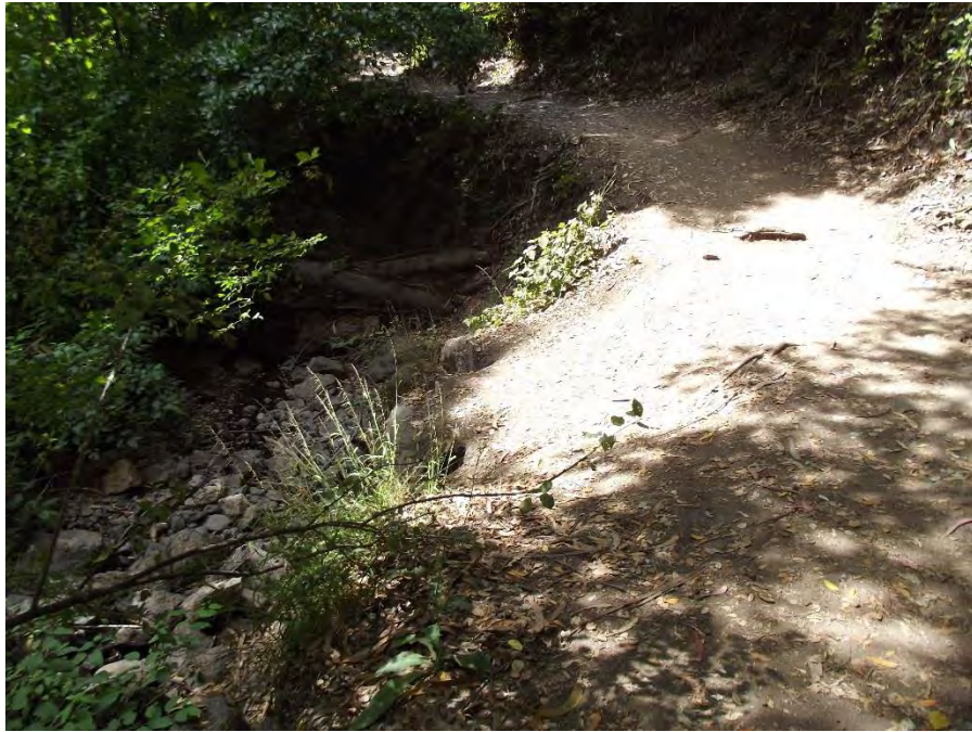
Location 17: Upstream from location 16. Water erosion is evident but the creek is also easily accessed from here, there is a fence both before and after this location—the fence should be connected and a retaining wall erected to discourage further erosion.
