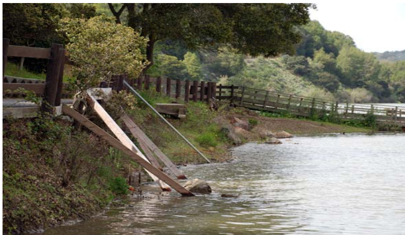
Eroded shoreline requires temporary reinforcement for walkway.
